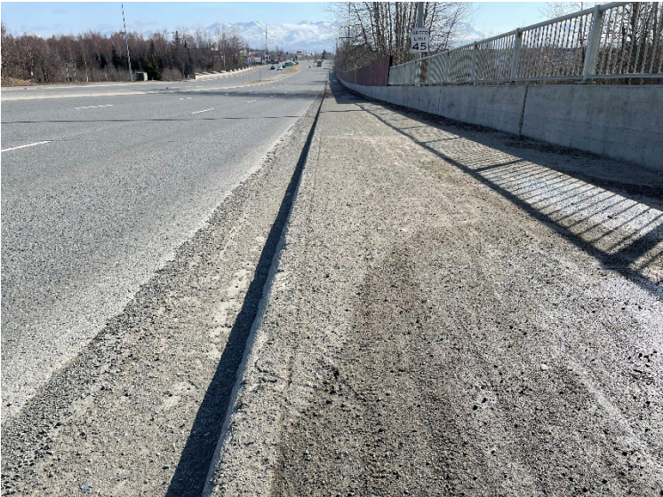
Figure 6.3 – Dimond Blvd before sweeping operations.
